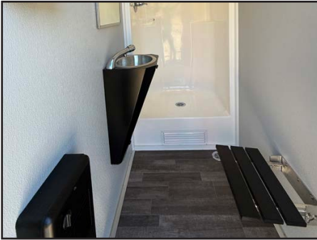
Each stall offers a shower, toilet or urinal, sink and a bench.
