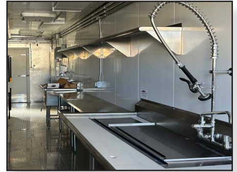
Three-basin sink and stainless steel tables with shelving.
