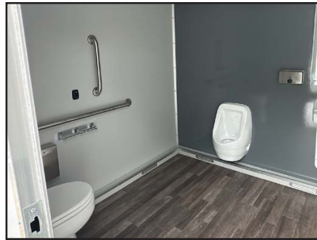
Waterless white urinals and toilets with ADA-accessible grab bars.
